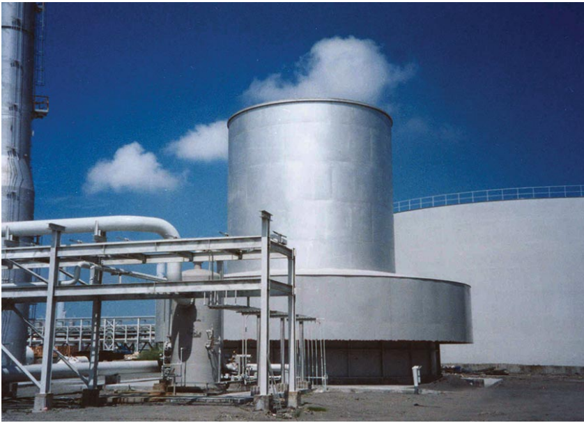
Enclosed flare (Image courtesy of Zeeco, Inc. ® – all rights reserved.)
