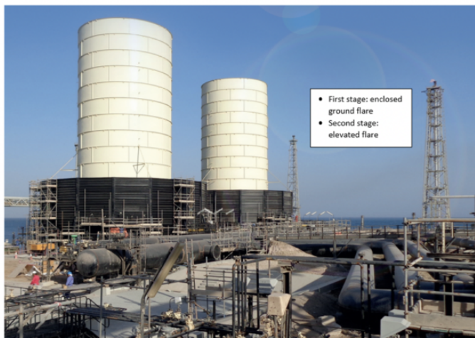
Figure 2: Example of a staged flare system consists of an enclosed ground flare (first stage) and an elevated flare (second stage)
